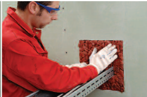
The foam expands after approx. 30 sec. and seals off the opening. No formwork required.
